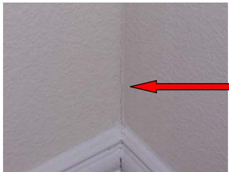
A crack was located in the mortar between two exterior walls located on the east side of the home.
