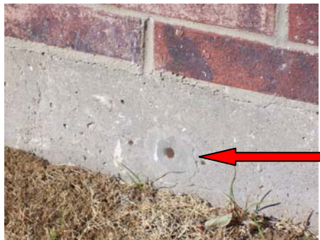
Exposed post tension cable ends were located on the north side of the foundation wall.
