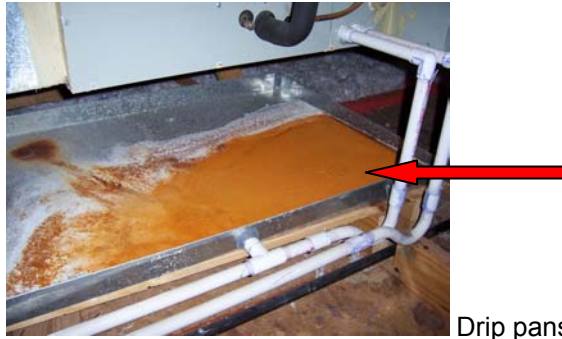
Drip pans located under the air conditioner unit are rusted from previous condensation.
