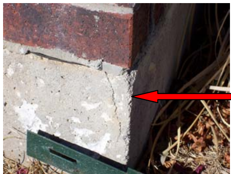
Spalling was observed on the west corner of the foundation wall.
